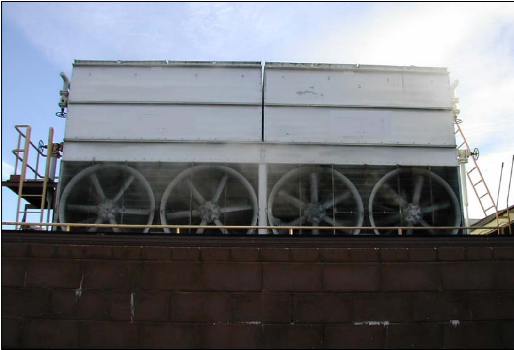
Figure 1 – Cooling Tower Before. (Haze Near Inlet Indicates Recirculation)
