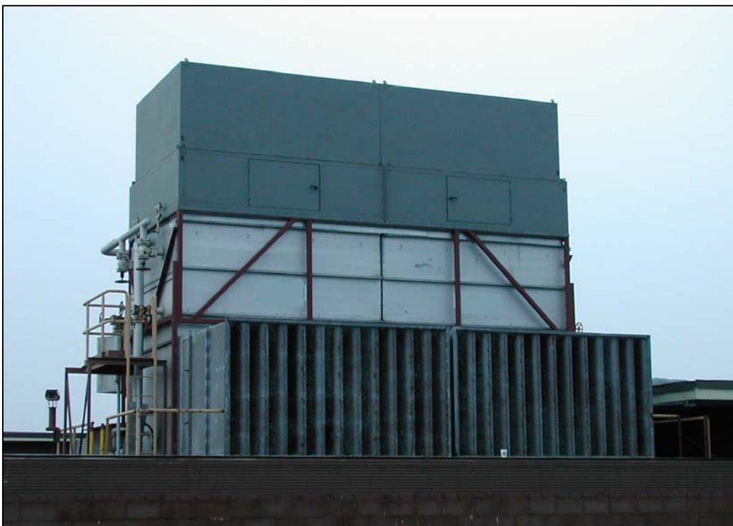
Figure 2 – Cooling Tower After.
