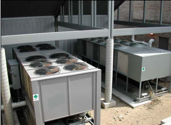
Dual Chillers Before Aeroacoustic Remediation, Complete With Recirculation Problems.
