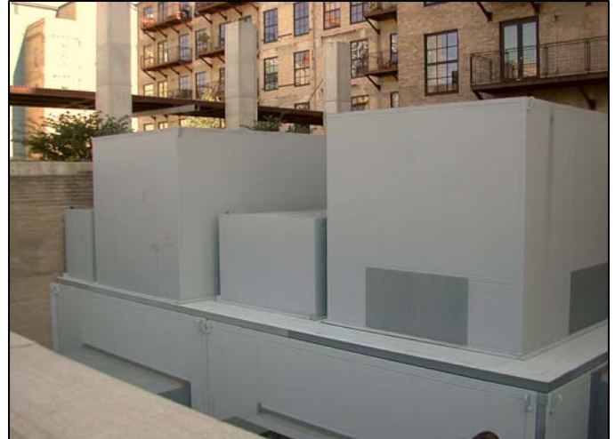
Dual Chillers After Installation Of Aeroacoustic Enclosure Flowing Approximately 300,000-SCFM
