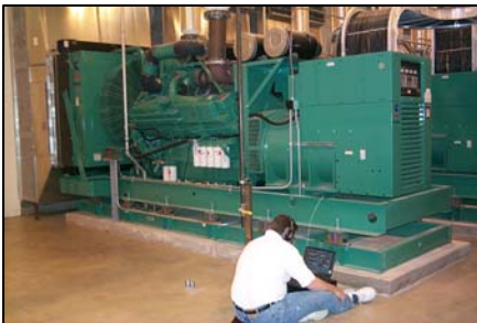
Vibration: Dynamic Transfer Function Analysis & Seismic Measurements
